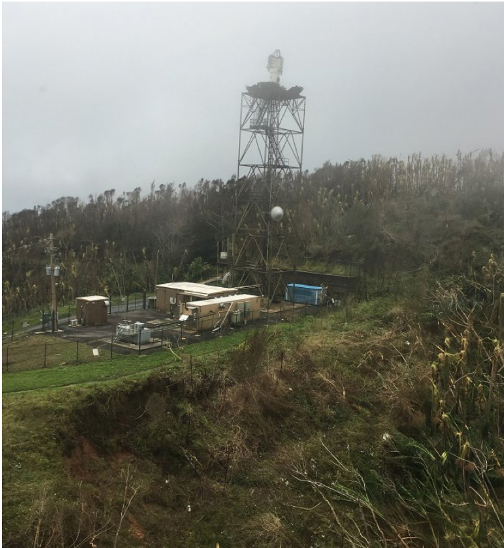
Damage to NWS San Juan's Doppler Radar in Hurricane Maria. Picture by Ernesto Morales (NOAA/NWS).
